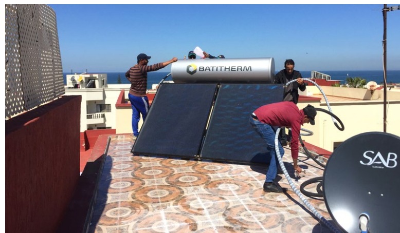
Technicians install solar panels on the roof of a house in Rabat, Morocco, April 2021.
